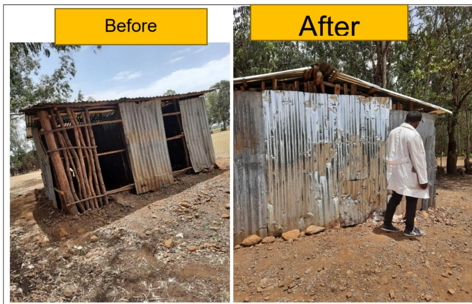
Figure 27 Latrine rooms built after CSC Implementation and action plan in Kidist Hana Kebele
