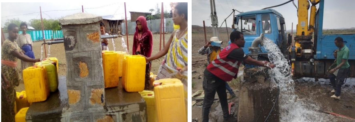
Figure 3: The community fetching water from the solarized water schemes in Guhalla; and pump testing after the installation of the solar-powered water schemes.
