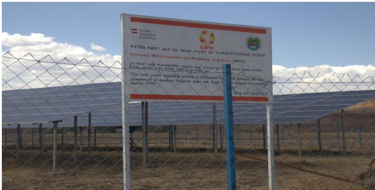
Figure 2: Solar-powered water system at the borehole - 10.5km away from the town.
