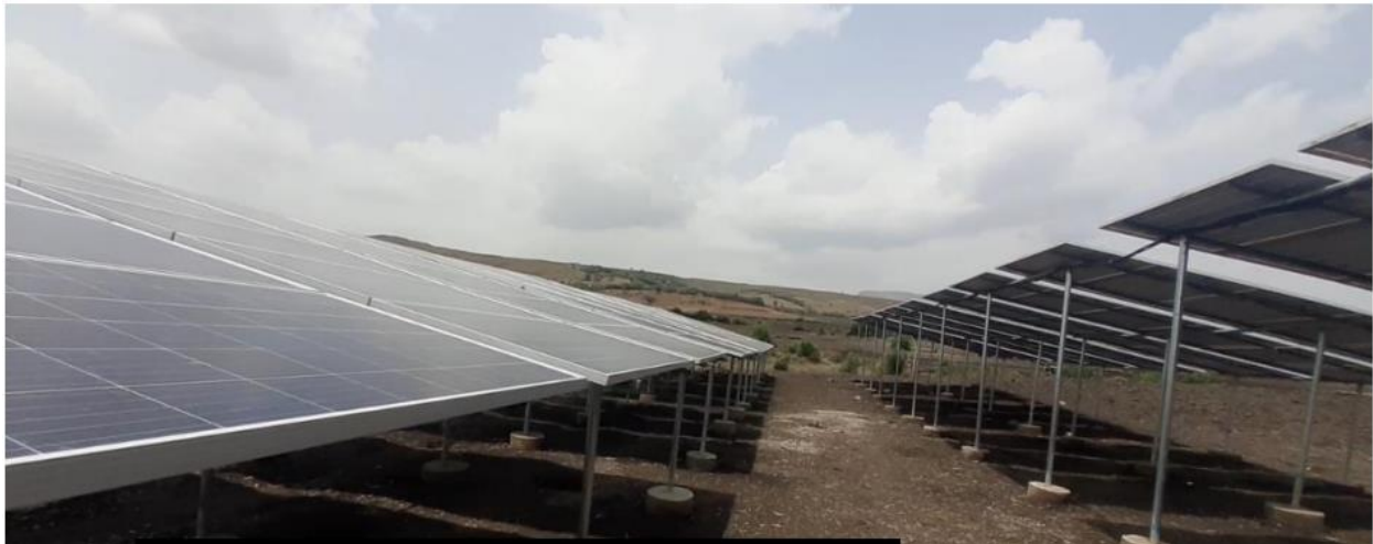
Figure 6: Installed solar panels (Baja Ferfer water supply scheme)
