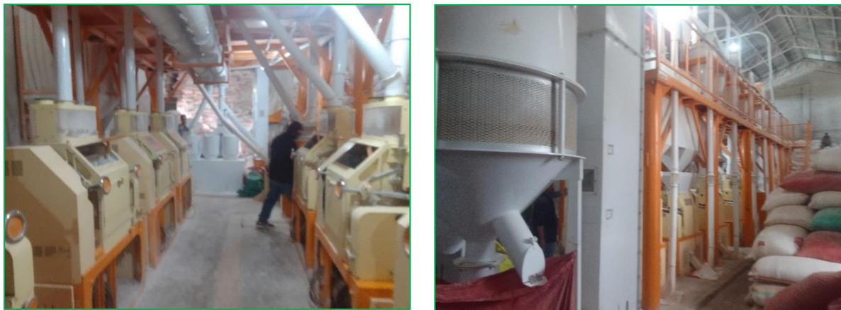
Figure 1: Limalimo Wheat Flour Factory; a potential market outlet for local wheat producers.
